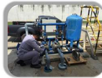
Booster pump service
